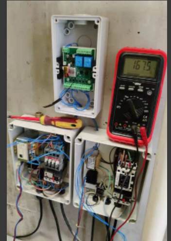
Tether installed on the stormwater pump in carpark located in a waterproof enclosure
